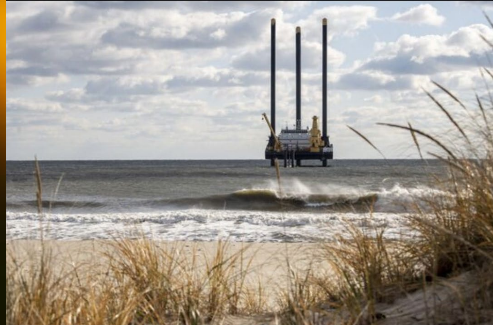
The construction of a wind farm off of the coast of Long Island near Wainscott, New York. Photographer: Johnny Milano/Bloomberg
